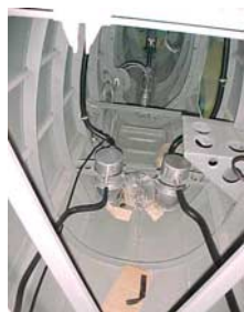
4 - Neutral gas plumbing
